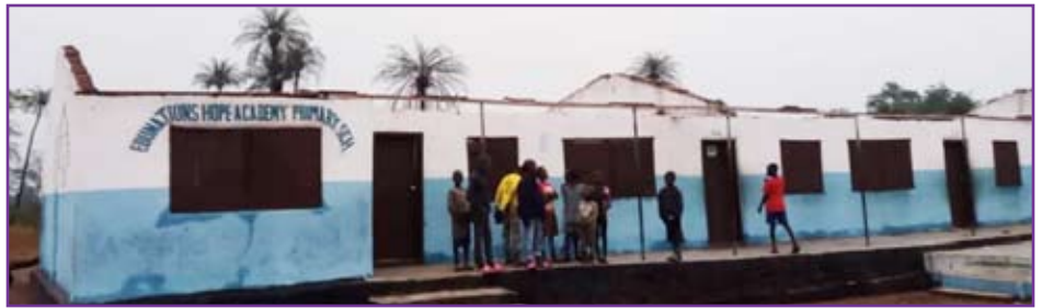
A large storm tore off the school roof in Mayatta, Sierra Leone.
